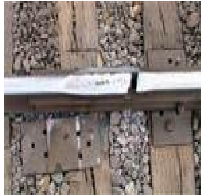
(Fig7.1Detection of cracks)
